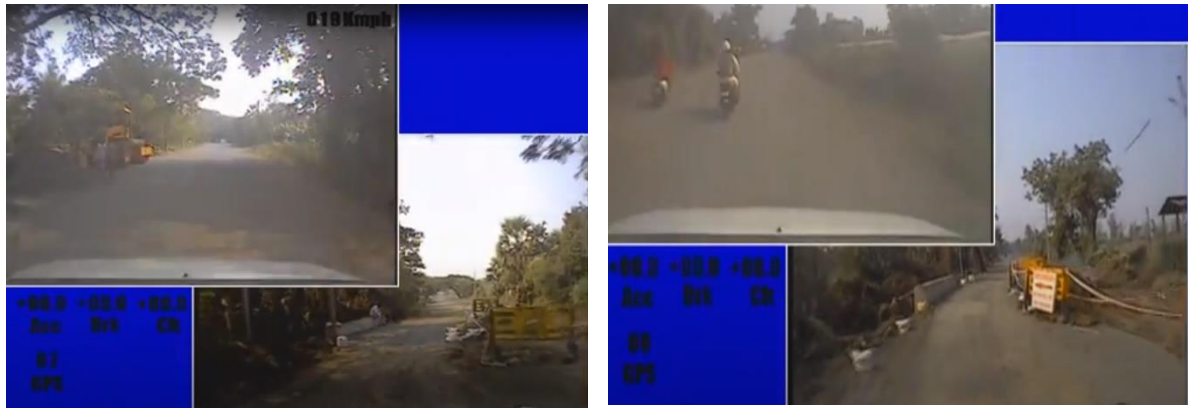
Figure 3.4 SH 31, Chinchani- Vangaon section of road in deteriorated condition
